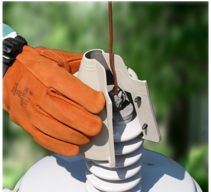
Figure 20: Example - Wildlife guards on overhead equipment
