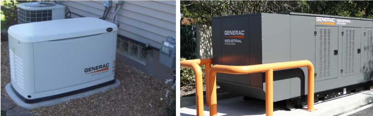
Figure 45: Example Residential and Commercial/Industrial Natural Gas Generator Sets
