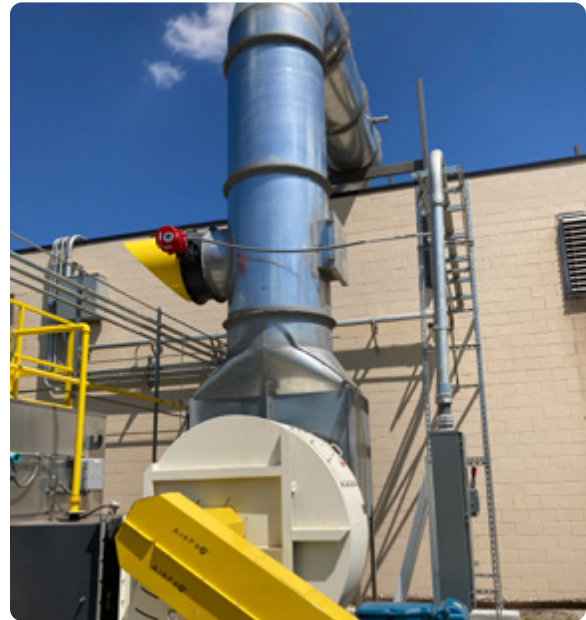
Newly Weds Foods' regenerative thermal oxidizer will reduce fuel consumption and improve efficiency
